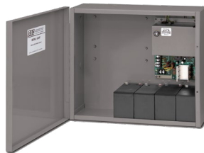
634RF with (4) optional backup batteries
